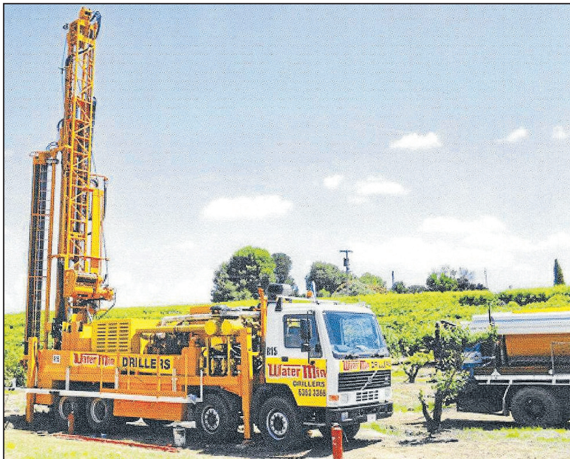
Watermin Drillers offers over 50 years operational experience designing and drilling water bores.
