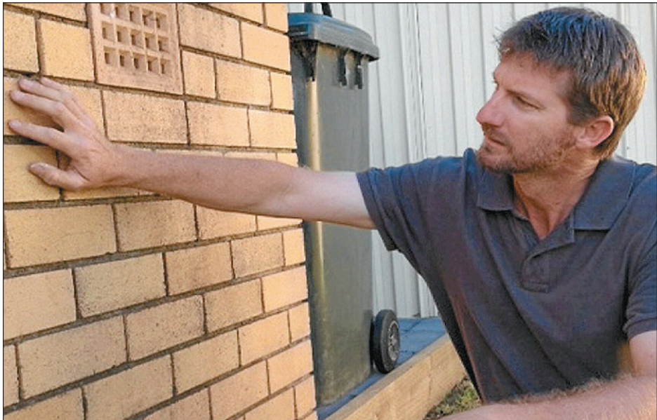
CHECK FIRST: SBC Building Inspections' Pete Ward undertakes a pre-purchase building inspection.
