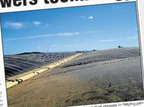
EFFICIENCIES: The 115 metre long pond has a dual purpose in helping generate energy and in providing organic fertilisers for Blanyre Farms.
